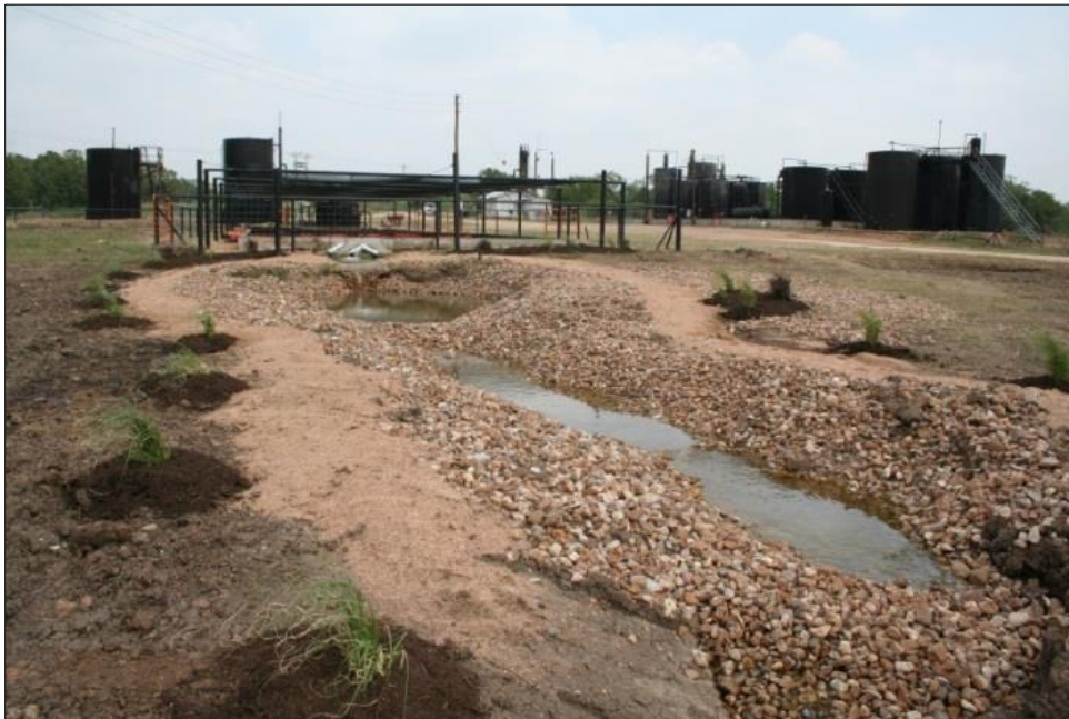
Fresh, Produced Water Outfall
